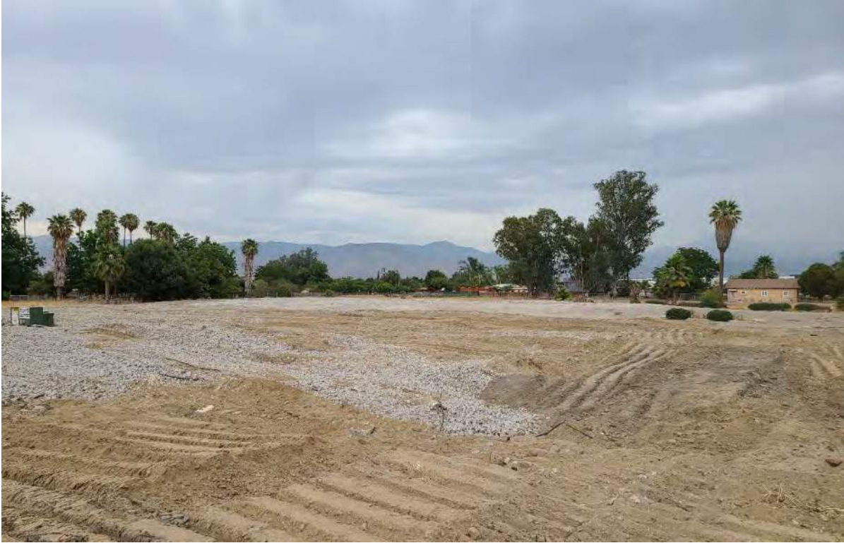
Figure 5-1. Overview of demolition debris in APN 0280-121-47, looking northeast.
